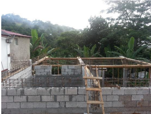
Ideal Christian Fellowship's new church foundation. Far from finished but we are trusting God for His provision.
